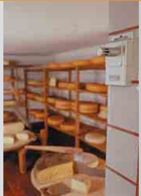
Monitors humidity and temperature in storage rooms
