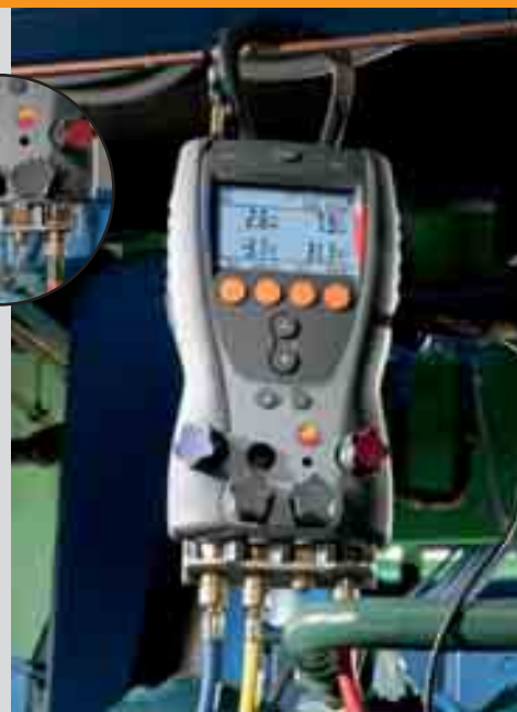
Measurements on a heat pump
