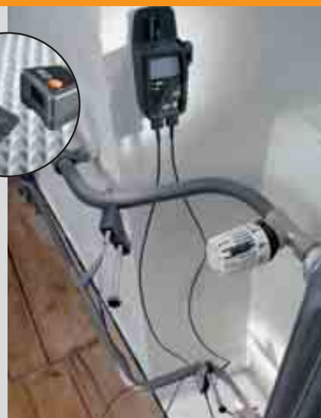
Inspects flow/return temperature
